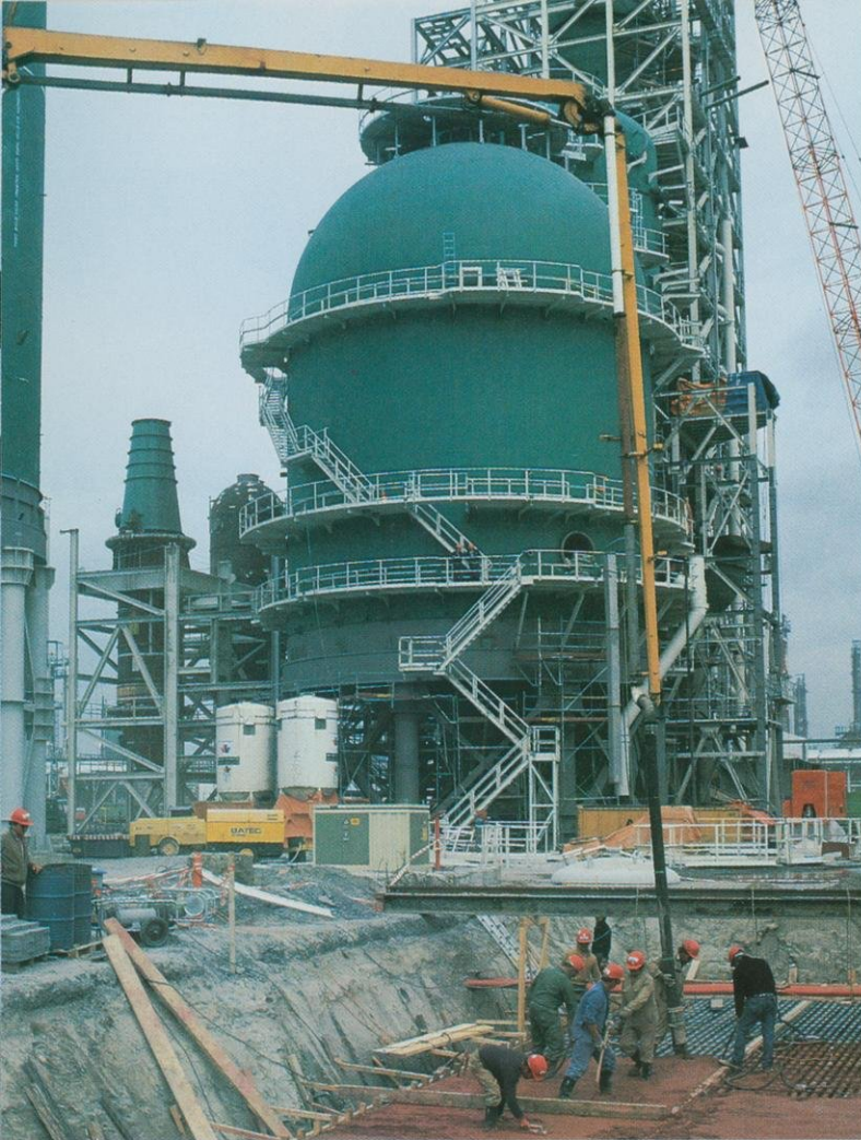
Workers at left are preparing the foundation for the FLEXICOKING unit which is part of a $560 million upgrading project at the Rotterdam refinery. The unit, which uses an Exxon-developed process to convert heavy fuel to light products and fuel gas, is scheduled to start up in 1986 at a rate of 32,000 barrels a day. A similar installation under construction at Baytown, Texas, will go on stream in 1987.
