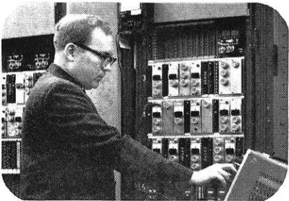
INDUSTRY CONTROL engineer Bob Vaughn, Virginia Polytechnic Inst., worked on drives, control and the new SCR armature regulator, from design through installation.
