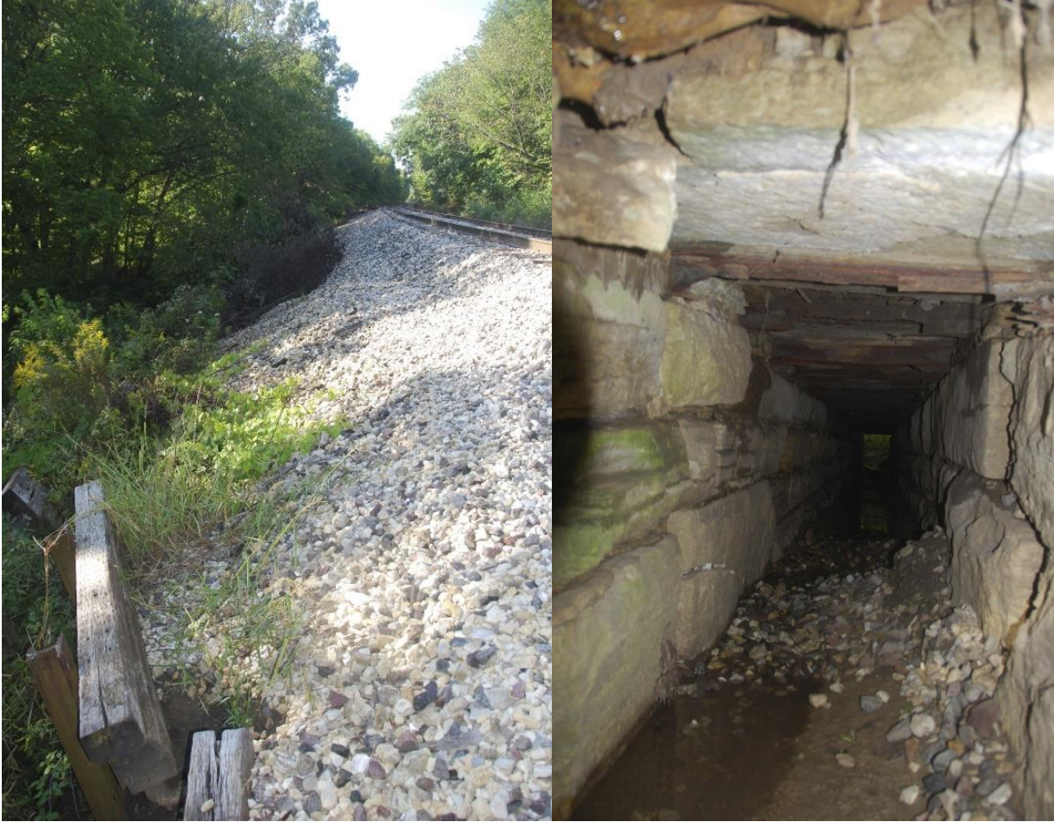
Figure 3.10 Culvert Site. Note Ballast Washout and Culvert.
