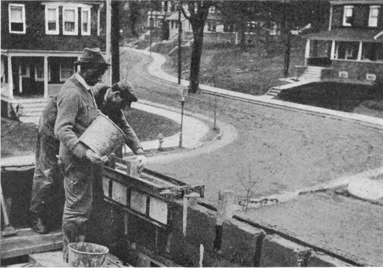
BUILDING A HOLLOW CONCRETE WALL: THE SPACES LEFT IN THE INNER WALL ARE FOR THE INSERTION OF FLOOR JOISTS.
