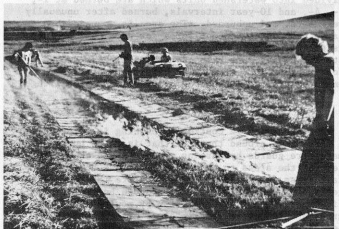
Fig. 2. Method of burning fire guards. The fire is being started with a drip torch by the person at the right as the metal strips are pulled along. The band of chain usually prevents the fire from burning under the metal. One worker with a fire swatter and another with a hose from a power pump on an all-terrain vehicle are ready to extinguish any fire left behind the metal strips.
