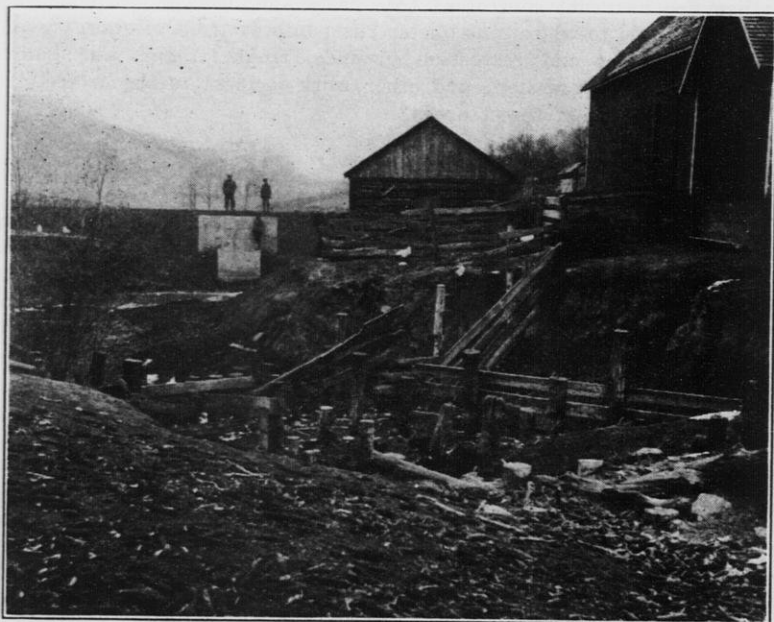
A typical soil saving dam. Note that the gully threatened even the farm buildings.
