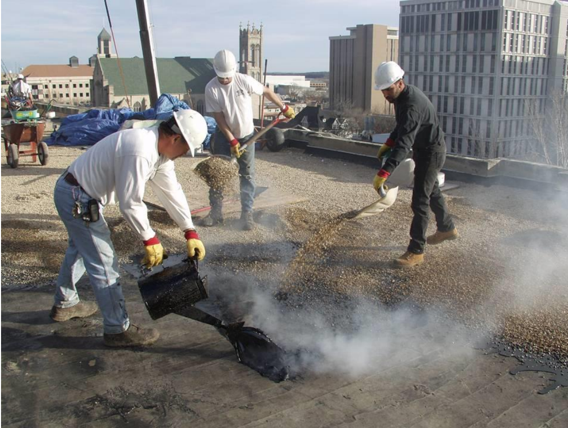
Photo 1-1 – A BUR roof system being installed on Chamberlin Hall on the University of Wisconsin - Madison campus.
