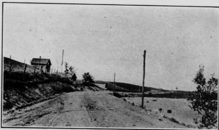
Typical Northern Wisconsin State Aid Work, town of Pike Lake, Oneida County.
