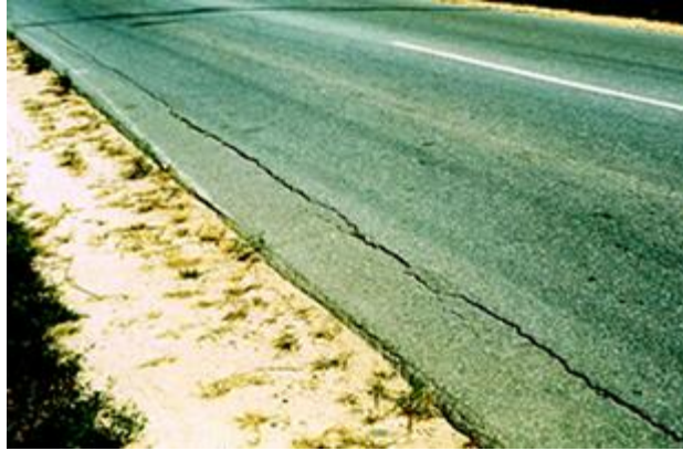
Figure 15: Longitudinal fatigue cracking in asphalt pavement
