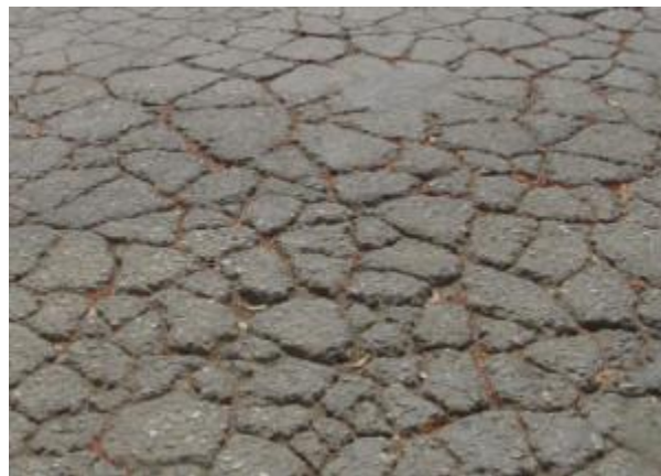
Figure 14: Alligator fatigue cracking in asphalt pavement
