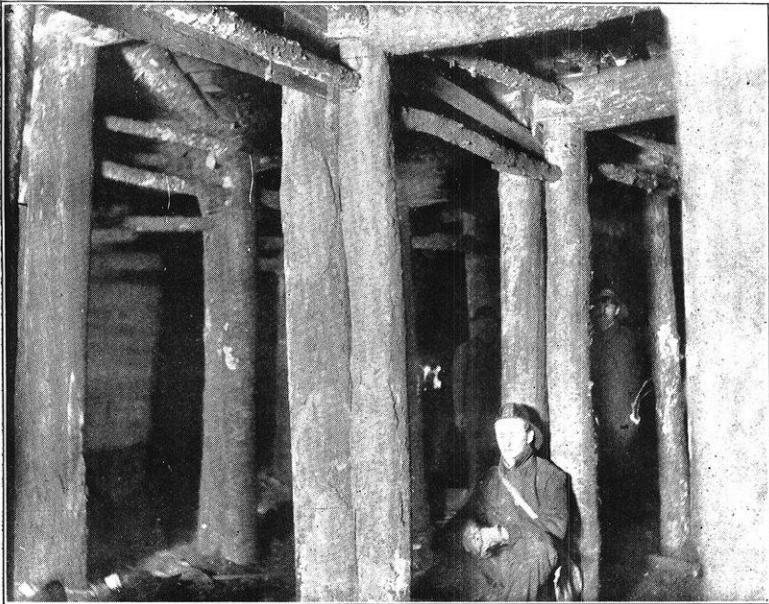
Timbering slice-sets. Note spags from posts to post and cap to cap.
