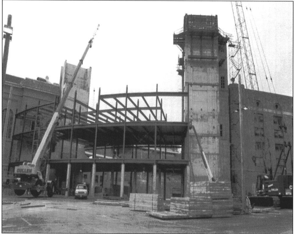
The steel skeleton of the new section in the south endzone at Camp Randall.
