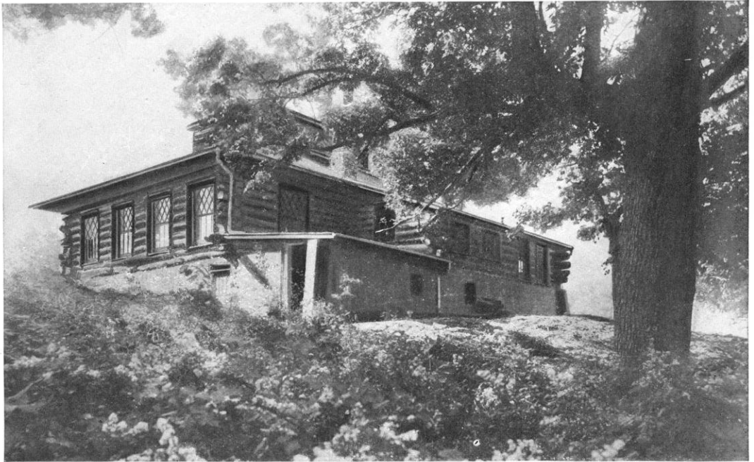
BOYS OF THE INTERLAKEN SCHOOL BUILDING THE LOG GYMNASIUM: THE SIXTH DAY OF THE WORK. A LOG AND CEMENT HOUSE BUILT BY THE INTERLAKEN BOYS.
