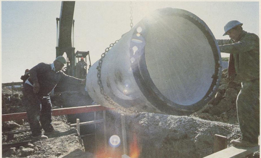
Preplanning and early installation of utilities avoids continual exposure of raw ground, cuts down on sediment and runoff.
