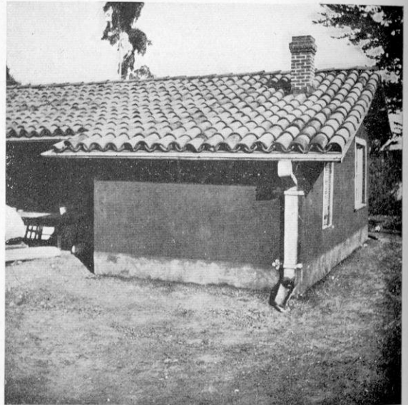
AN OLD MISSION TILED ROOF LEFT TO THE DESTRUCTION OF TIME. THE OLD TILES ARE ILL AT EASE NEAR A SMOOTH MODERN ROOF. SHOWING THE IRREGULARITY OF THE OLD HAND-MADE TILES.
