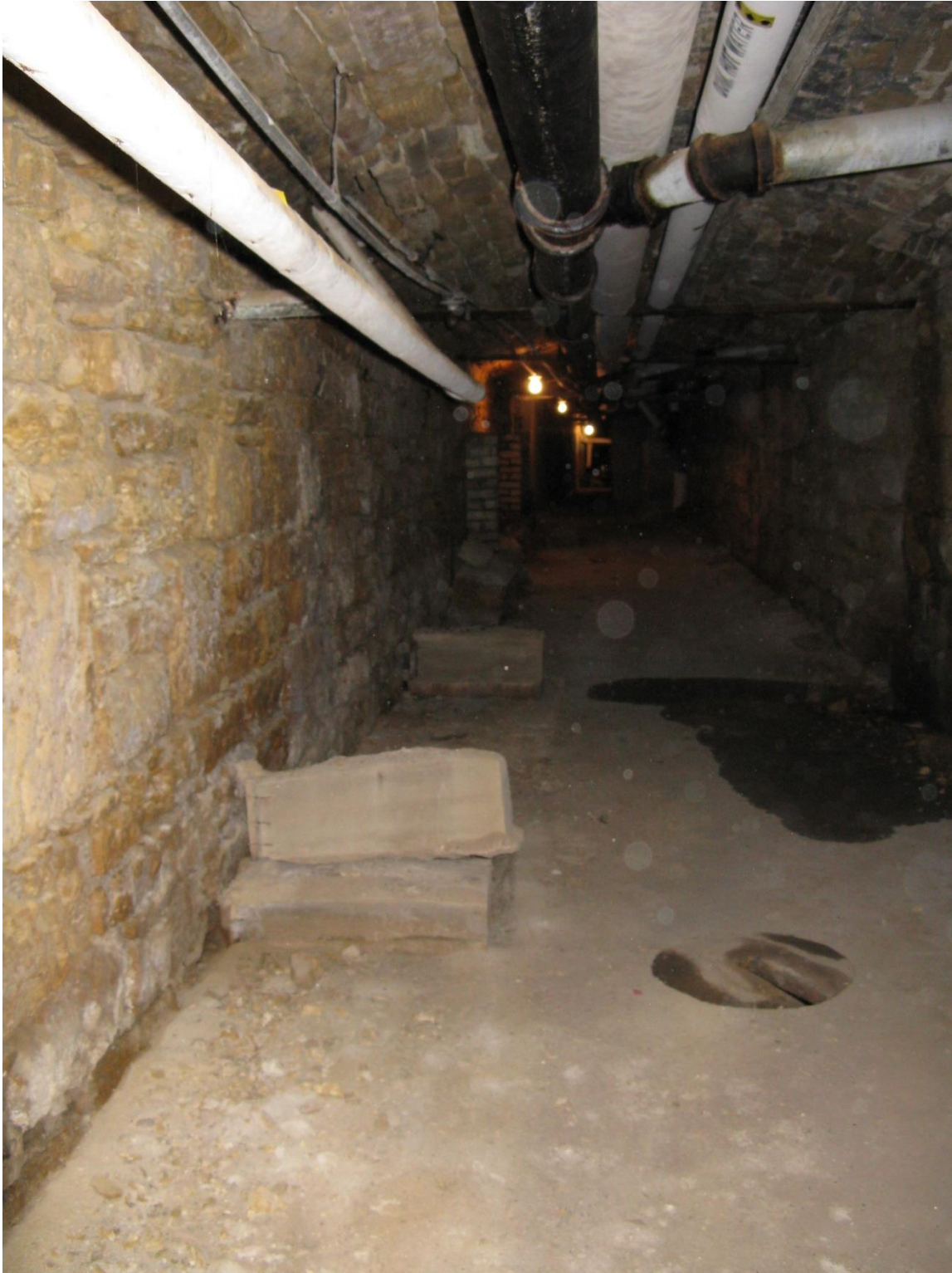
Figure 2.36. Utility tunnel running east and west beneath Center Main. The end of this tunnel connects to the higher level common tunnels that run north and south. (Photo by the author, 2007)
