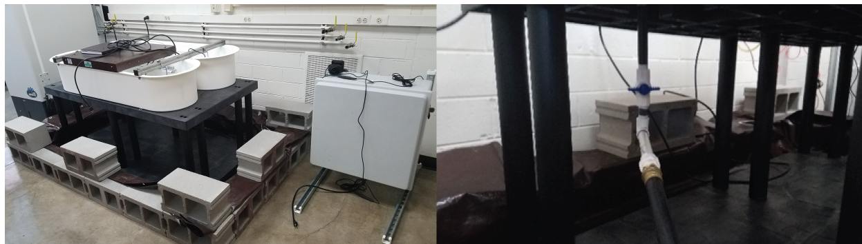
Figure 55: Left: The early ORP constructed within a retaining wall. The retaining wall acts as secondary containment in case there is a spill. Right: The plumbing system beneath the ORP is shown. This drainage allows for easy draining of the ORP after use or during cleaning.
