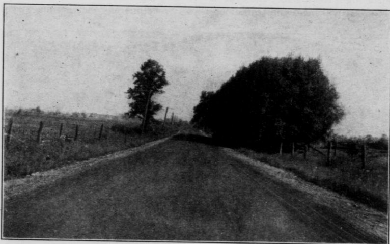
Cedarburg Plank road, Town of Mequon, Ozaukee county. 15-foot gravel base with crushed limestone top. Built in 1914; surface treated in 1915 and again in 1916; showing the effect of persistent maintenance. This road is subject to very heavy traffic, as it joins one of the Milwaukee county's main concrete highways, and is standing up exceedingly well.
