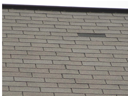
Figure 7.1: An example image from a roof survey that would get a positive reward for the “missing shingle” task in our experiment.
