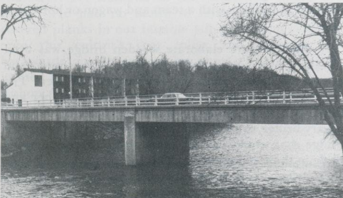
Present bridge was built in 1924. Original concrete railings have been replaced by new steel bars. Building in background is Riverview Apartments, village operated housing unit.
