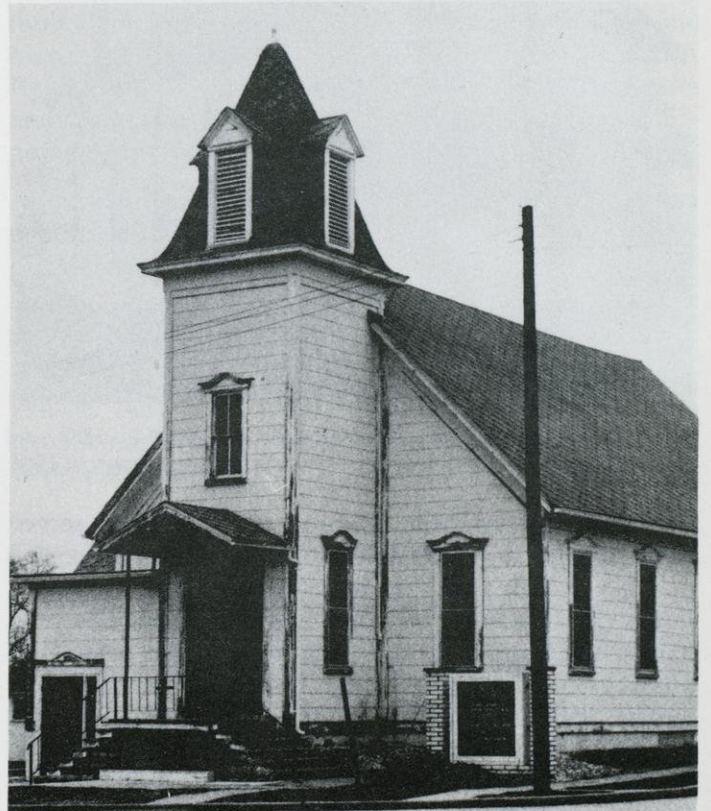
Baptist Church as it appears today. Exterior of the church was being repaired and painted when photo was taken.
