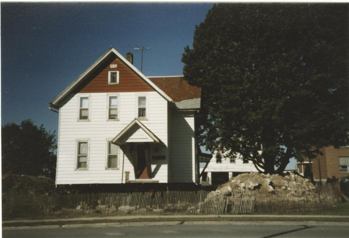
The house is readied for removal from the property for school expansion in September 1988.
