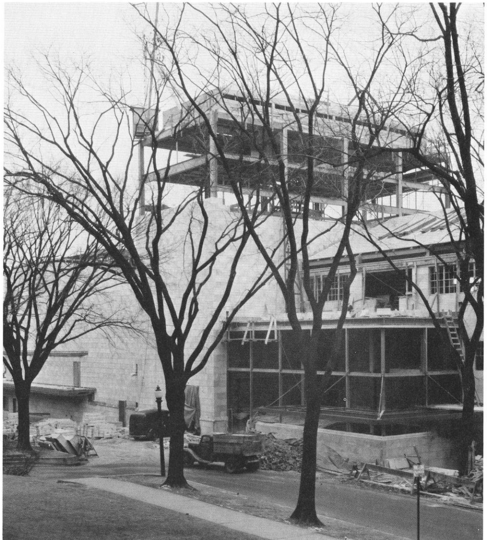
The new theater wing rises on the west end of the building in 1939.
