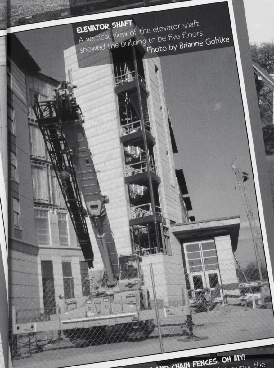
THANKS TO MIRON Miron Construction served as the general contractor of the construction project. Photo by Brianne Gohlke
