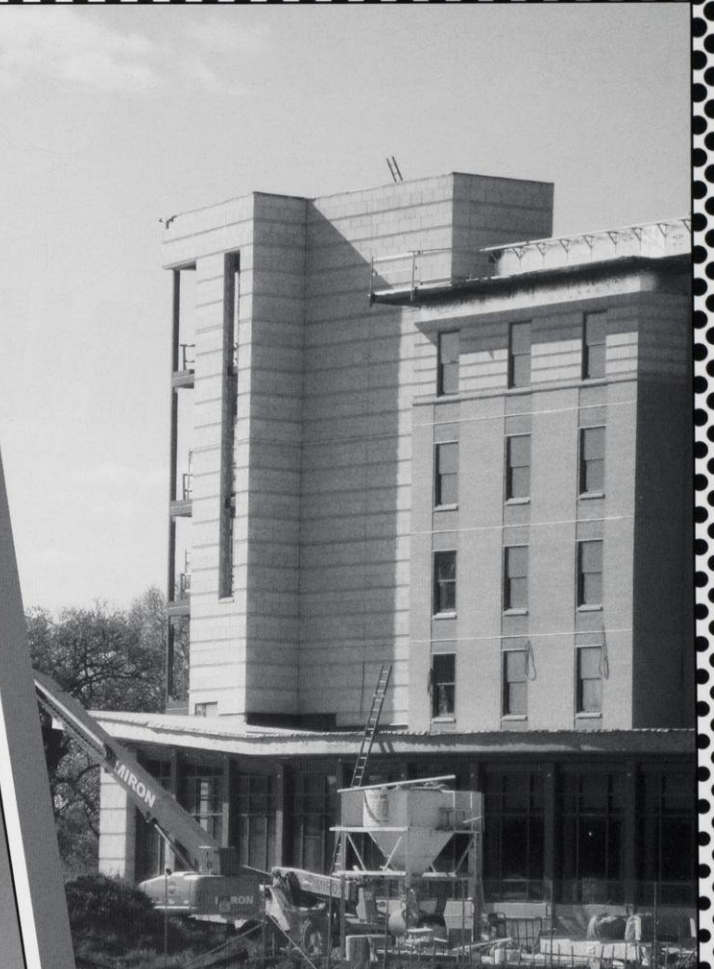
SERVICE WITH A CAPITAL 'S' The new Lakeshore dormitory featured a new dining service facility, which was estimated to serve more than 1,300 daily. Photo by Brianne Gohlke
