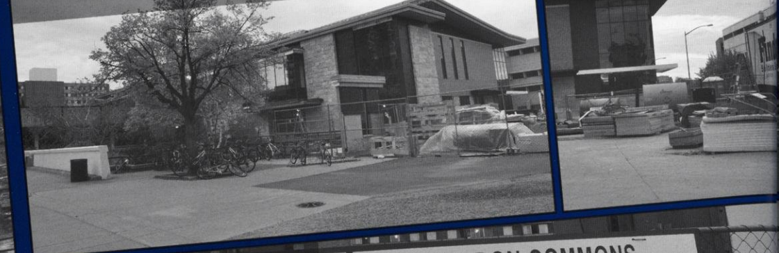
CONSTRUCTION SITE Even on a cloudy day, the new addition to Gordon Commons shimmered with beauty. Photos by Bretta Schmidt
