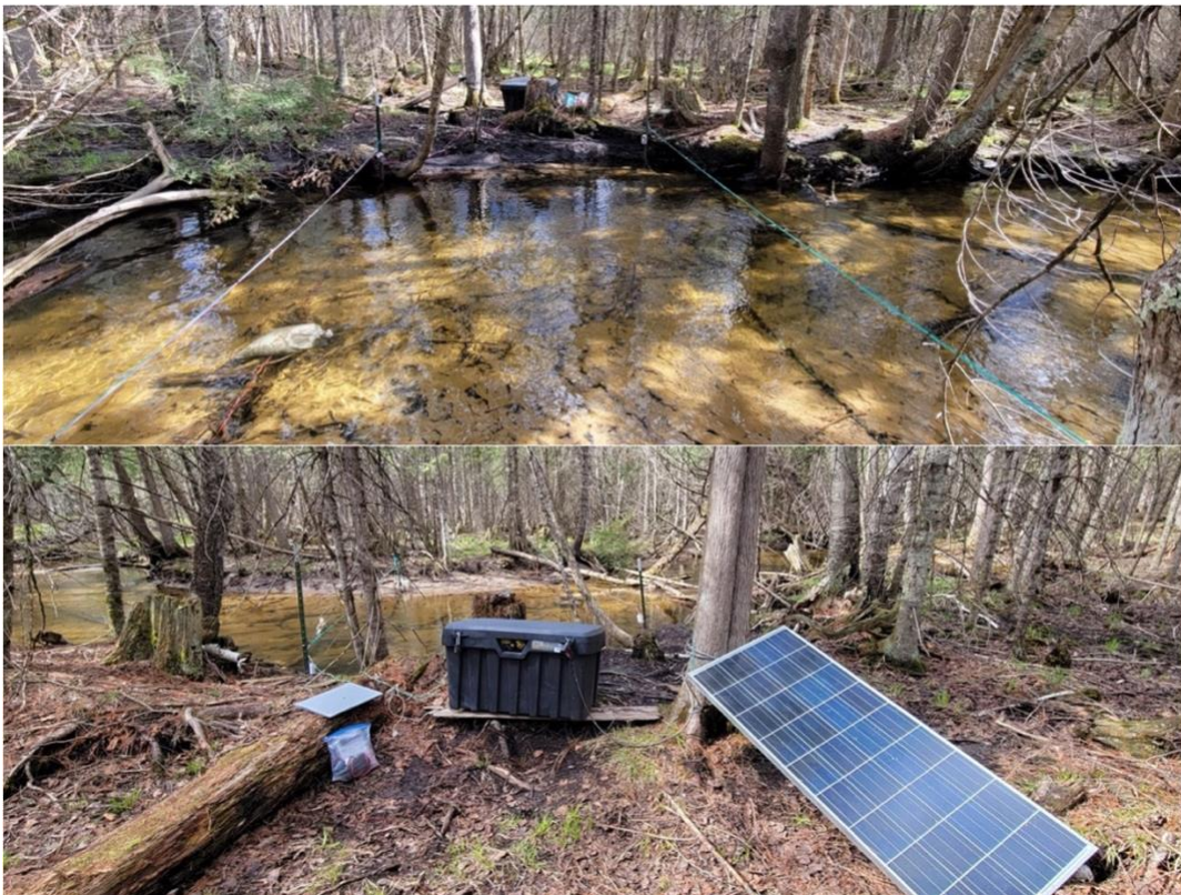
Figure 5: With permission from the landowner, we installed the Lower Nejedlo PIT array downstream of the road crossing. Image of the Nejedlo PIT monitoring system from both the right bank (top) and the left bank (bottom). Image shows the set-up and antenna placements.
