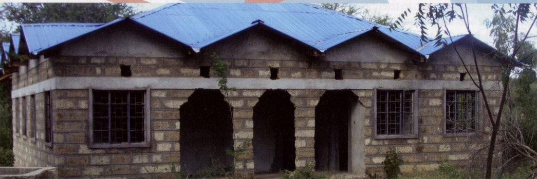
Lesley Sager is working closely with the village leaders of Gutanga to convert this unfinished building into a Makerspace.
