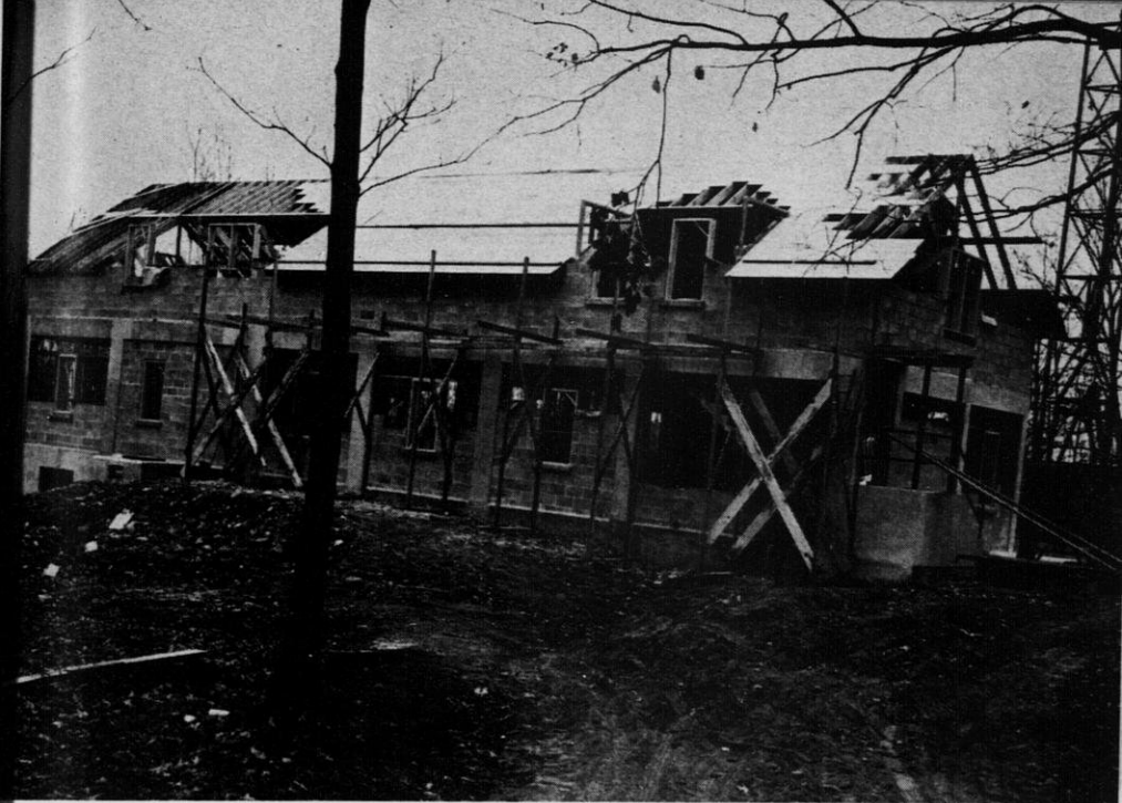
Cornell ranger station under construction. Design of structures is part of the engineering division's work.
