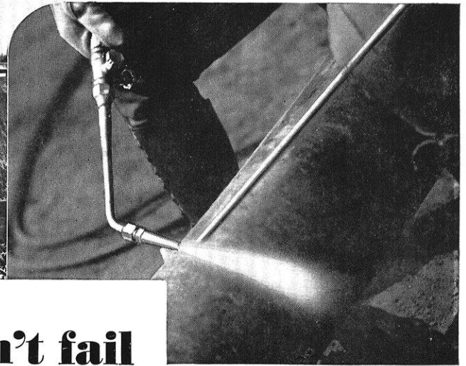
Two 10-in., one 14-in., and one 6-in. lines were laid on this trestle. Insert shows close-up of Multi-Flame Lindeweld Head in action.
