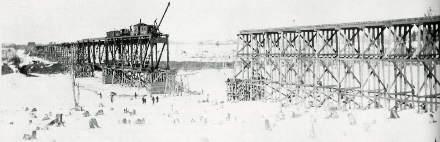
Construction crews were nearing completion of the Wisconsin Central Railway bridge across the Flambeau River in Ladysmith in the winter of 1906. The trestle was one of the longest on the line. This view looks north.
