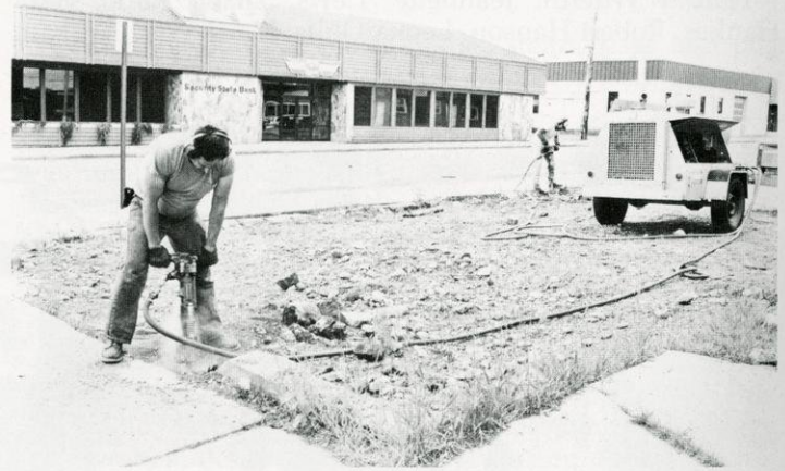
Earl Monnier and John Holm of the city crew chipped away the foundation of the old Grooms building as work began on Centennial Square, located on land leased from Melinda Olsen and Catherine Gouze.
