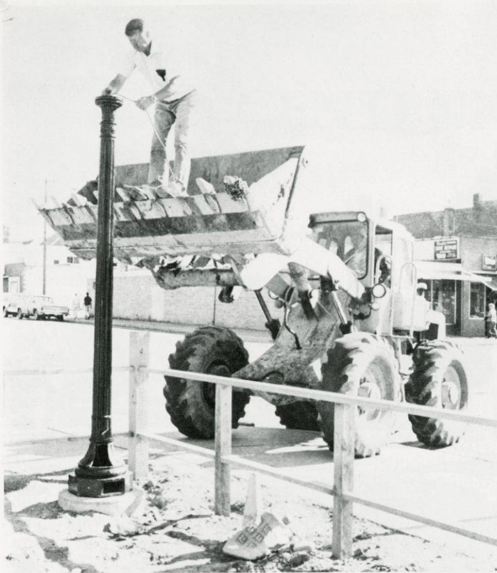
Jerry Selvig adjusts a wire in an old city street light incorporated into the design of Centennial Square.
