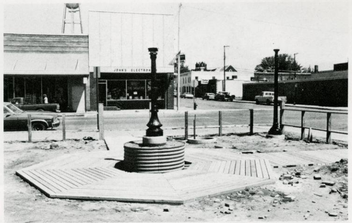
The octagon boardwalk around the central light pole and planter was completed and the site was ready for leveling. The county donated a culvert which was used as a planter.
