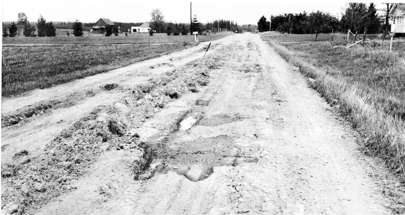
Figure 21 FROST HAZARD ACTION
