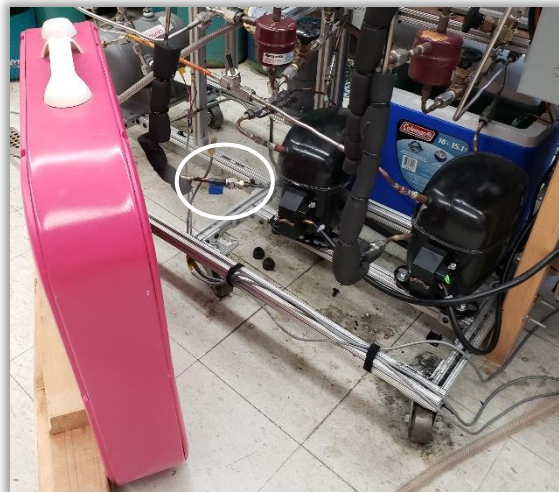
Figure 8.9. Photo of fan for compressors.
