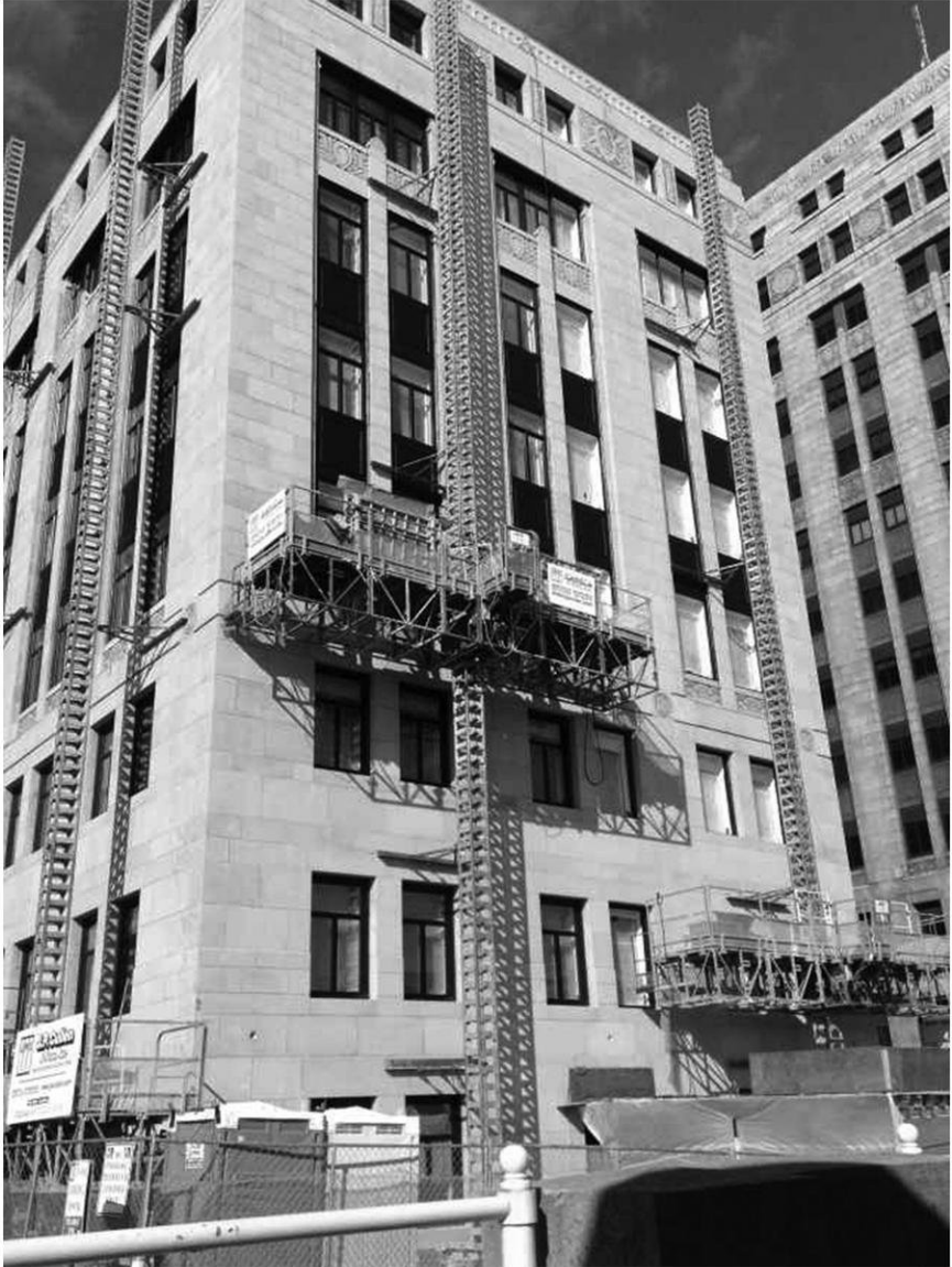
The Department of Health Services building undergoes window replacement in 2013 as part of a $14.5 million, 18-month, restoration project. Construction on the building, which is on the National Register of Historic Places, was begun in 1930, and is built of granite from the State Quarry in Amberg, Wisconsin. (Department of Health Services)
