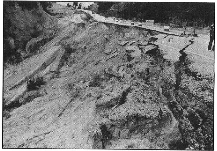
Poor service protection and drainage system lead to erosion and embankment failure on East West Highway in northern Malasia
