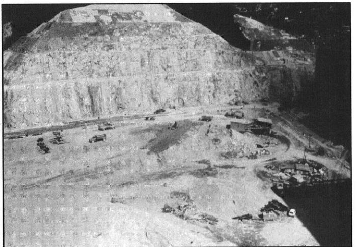
Clearing site in front of 150 foot high, 75 degree angle rock slope for building construction
