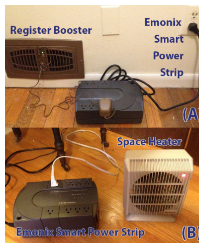
Figure 3.4: Photographs of our control equipment. (a) A register booster fan controlled by Emonix smart power strip. (b) An Emonix power strip controls a space heater that provides additional heat in rooms that are too cold.
