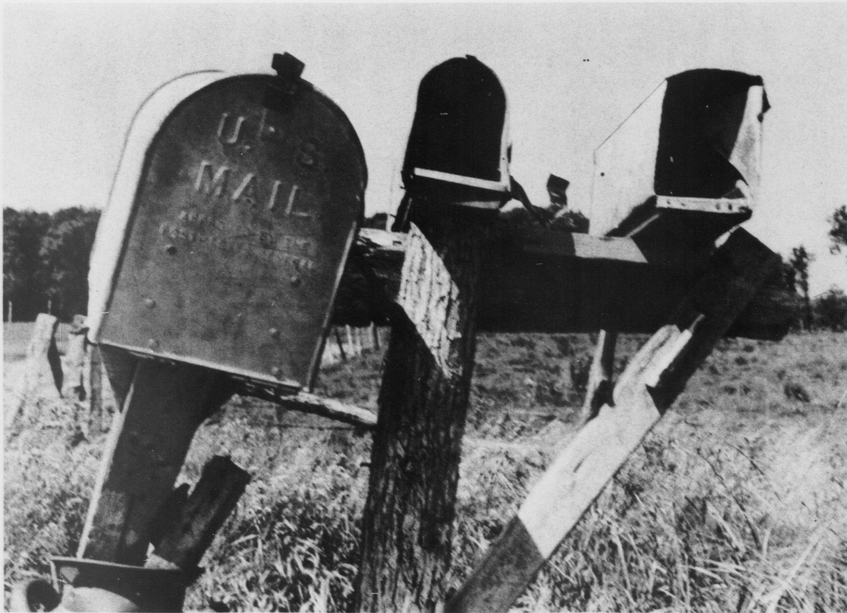
The problem that was faced in organizing and carrying out a mail box painting campaign is clearly illustrated in the picture. These boxes were found in Wood county.
