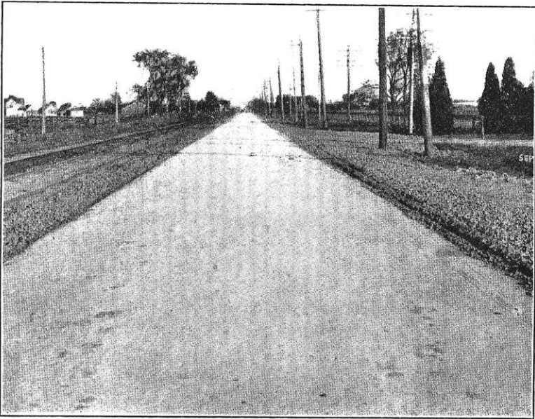
FIG. 5.—Grand River Road Three Months Later; 16-Foot Wide Concrete; 8 Feet of Gravel on Sides; Total Width, 24 Feet. Cost from $800 to $1,000 Per Foot of Width Per Mile.
