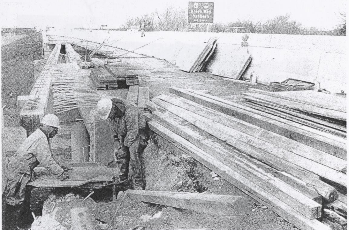
Workers expanding 441 bridge at the Tayco St. overpass, circa 1991. Menasha Public Library .
