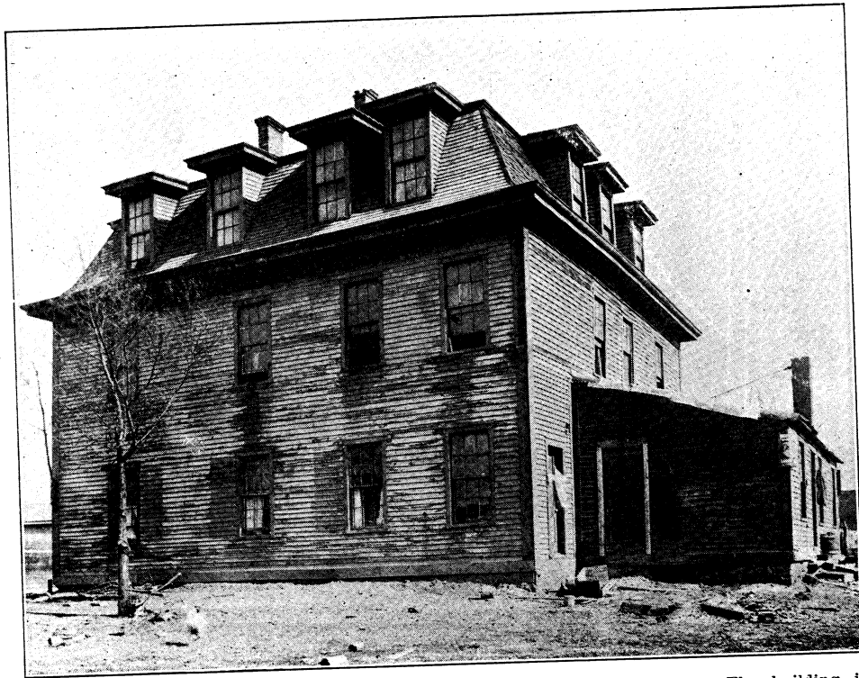
Illustration XIV.—Three story frame building occupied by forty-four persons. The building is structurally unsafe and without fire protection, plumbing or sewer connection. Between the time of first inspection and the time this view was taken the cornices had been patched, a trough taken in from a second story window, a new roof placed on the one-story addition, the basement boarded up and the front of the building painted.
