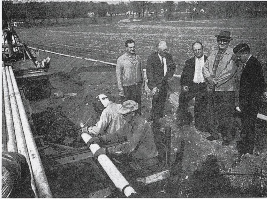
LAYING OF THE PIPELINE from Marshfield to Spencer, Wisconsin was inspected by Spencer Officials. Donald Putnam, Manager of Marshfield District, took the group on the inspection tour recently.
