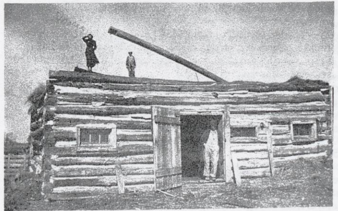
A building on the Wm. Gessert farm, wrecked by the wind March 27, 1938. Raymond is standing in the door and Marie is on top.
