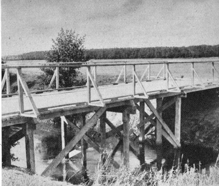
Completed bridge, built by US Army engineers for farmers of Harreshausen. Materials were supplied by village, and willing GIs got some practice in bridge-building.
