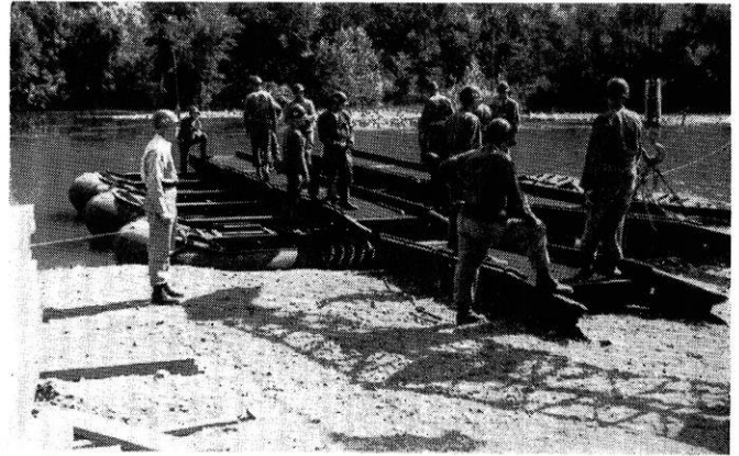
Cadets stand by as another section of steel treadway is lowered into place on a pontoon bridge.
