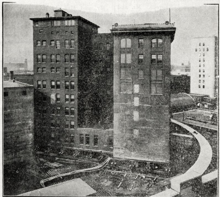
To arrive at a new location, the 8-story, 11,000-ton general office building of the Indiana Bell Telephone Company was backed up and then turned in a quarter-circle, without halting any of the normal activities within the structure. Elevators ran, gas, water, electric light and power, and steam heat were available as usual, and local and long distance telephone conversations continued uninterrupted. The move was to make room for new telephone building soon to be erected. Photo shows building with turn about half completed.
