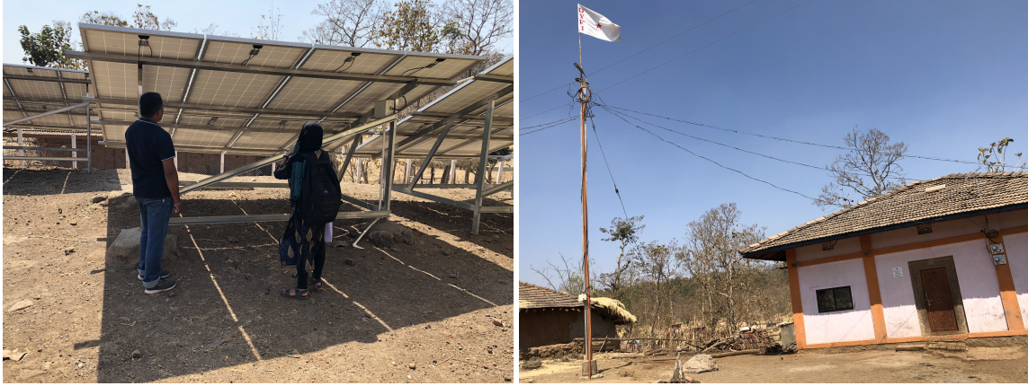
(a) PV panels
