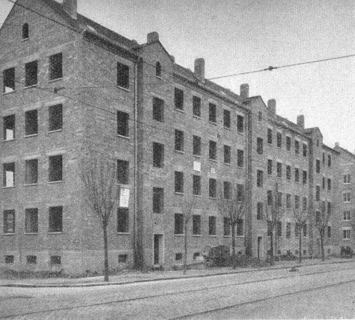
This uncompleted apartment house is to become home for 24 families. Project is being aided by a Marshall Plan contribution of DM 52,000 ($12,376), part of a DM 750,000 ERP allocation to help construct 286 family units in the area.
