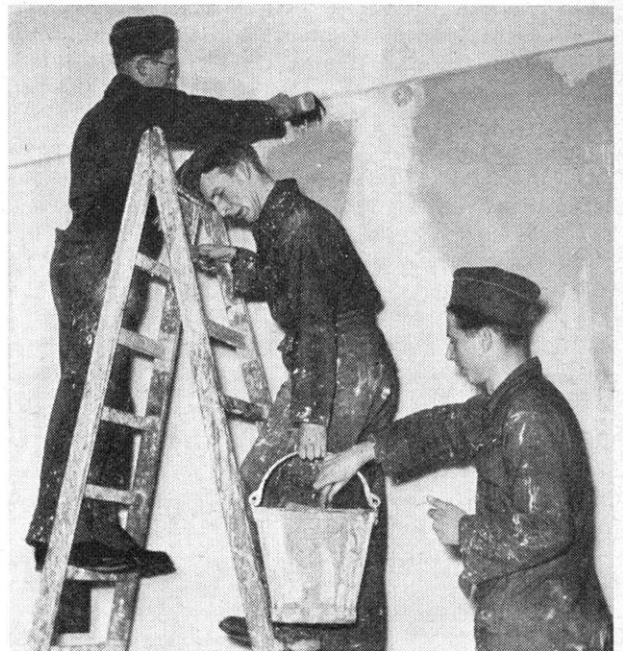
It's questionable where more paint is being applied: on walls or on dungarees of young volunteer workers making last minute preparations for recent opening of a new Neighborhood Home in Zehlendorf, Berlin. However, their efforts produced an attractive and much needed center which was partly financed by grant of DM 160,000 from HICOG Special Projects Fund. (PRB BE-HICOG photo)
