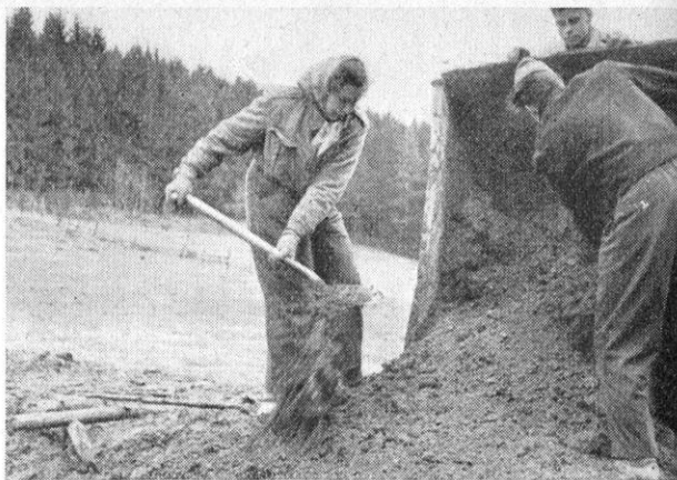
Ilse Fuercht from Bavaria lends a hefty hand in leveling ground for a Brethren Service playground in Germany.
