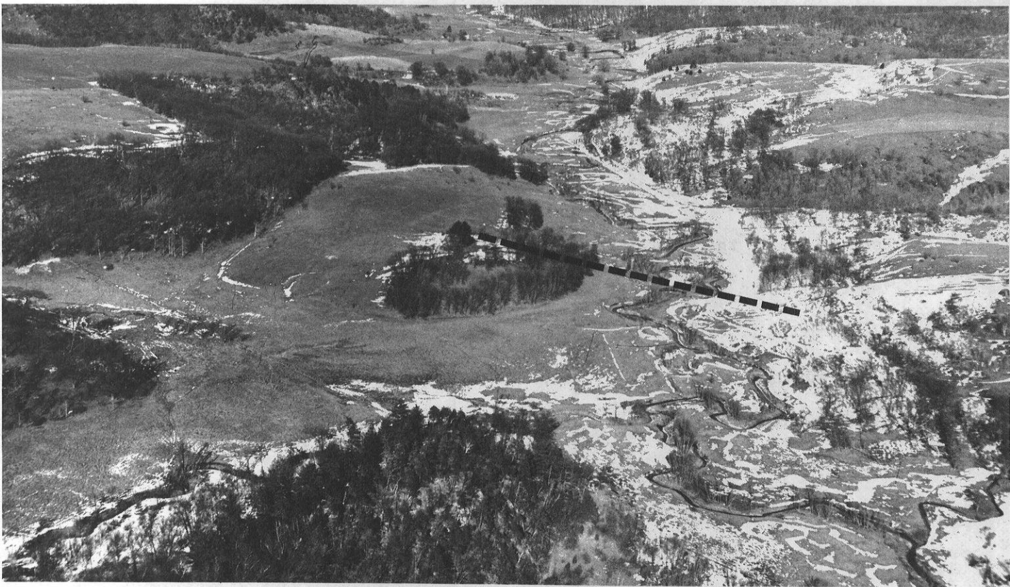
The Cox Hollow Lake basin before construction of the dike which is shown by the dotted line. When flooded, the North arm of the lake will extend to the left and the South arm will extend to the lower right. The impoundment will be drained by a spillway into the downstream channel which extends above the dike in the center of the picture.
