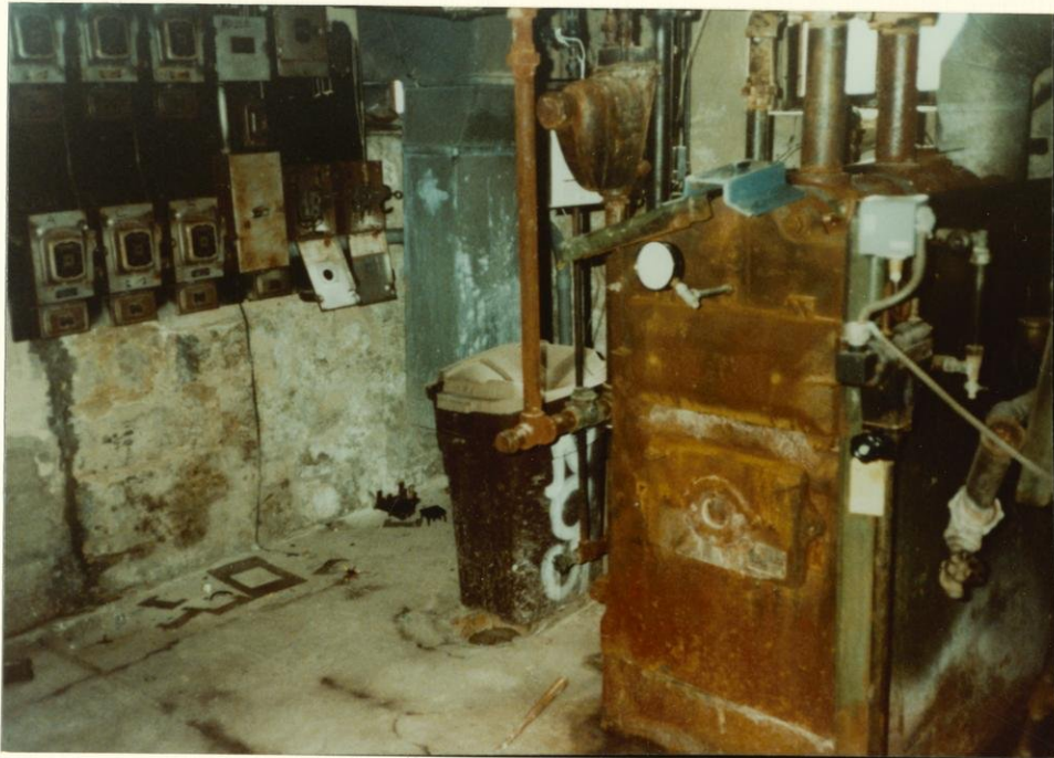
Basement - Heating System and Electric Meters
