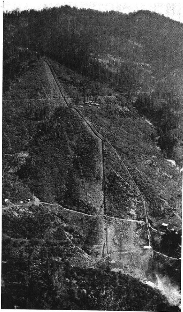
FIG. 6.— Power Drop No. 2. The Hoist Line Appears on the Right and the Penstock Line on the Left Terminating at Power House No. 2 Located on the Creek Bank. Construction Camps Appear at the Top, Half Way Down and at the Bottom of the Hill.
