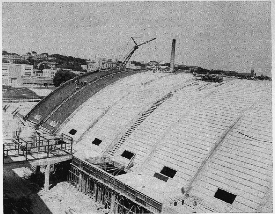
Grid fans this fall will see the Camp Randall Memorial practice building nearing completion.
