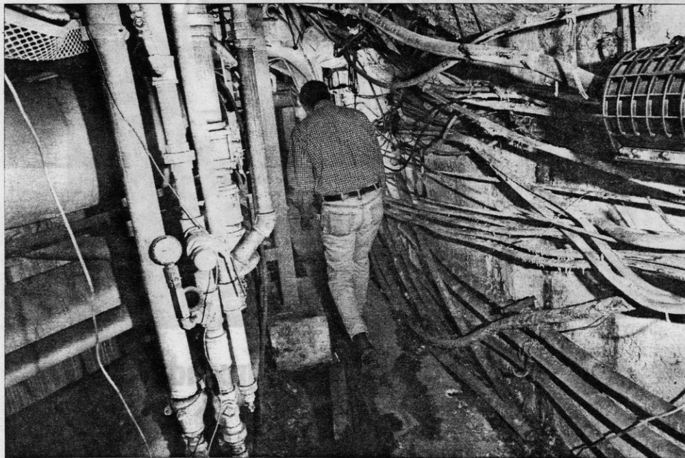
Physical plant steamfitter Les Breuning squeezes through a narrow space in an underground steam tunnel near the Charter Street heating plant. The dark,
