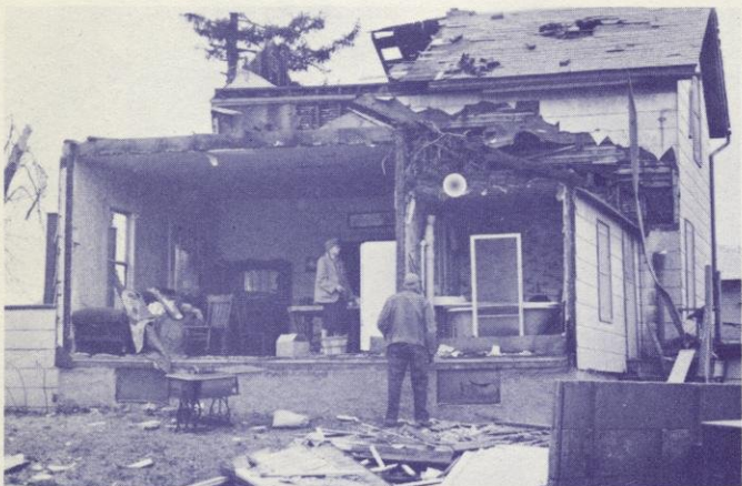
MONROE —Funnel literally exploded this home giving it the appearance of a lean-to.
