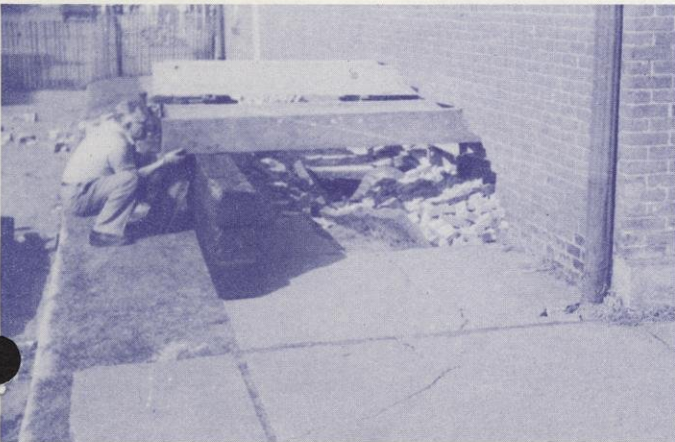
Corner of Klindt's Grocery in Cassville had to be shored up as its foundation was undermined by flood waters.
