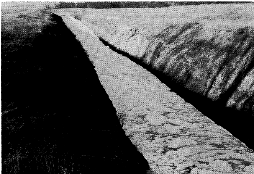
FIGURE 2. Ditch immediately below 54" pipe outfall. Note foam on water surface.
